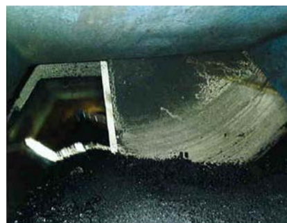
Cutters: these must cut the entire stream of material and be free of obstructions, intentional or accidental.
